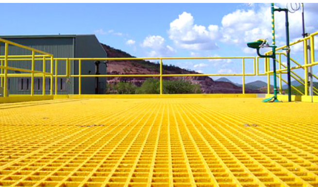
Corrosion resistant DURAGRATE® installed around the solvent extraction electrowinning (SXEW) process of a copper refinery in Piedras Verdes, Mexico.
